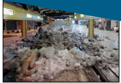
Costly. Before the installation of the Nordic systems. Several tons of ice to de-ice. It will take several hours before the train is back in service.
