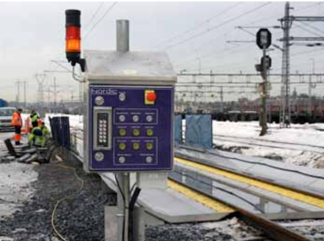
Operating panel by the track.
